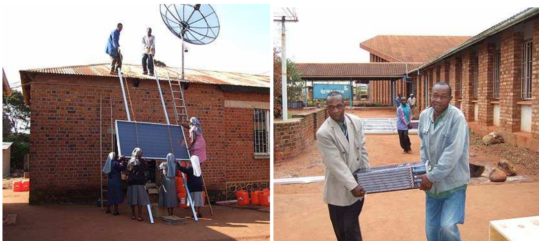
Fig. 5.8: Low-tech hoisting of PV Module and transport of Lead Acid Batteries at the Mbinga Sisters’ Convent (southern Tanzania) [52]
