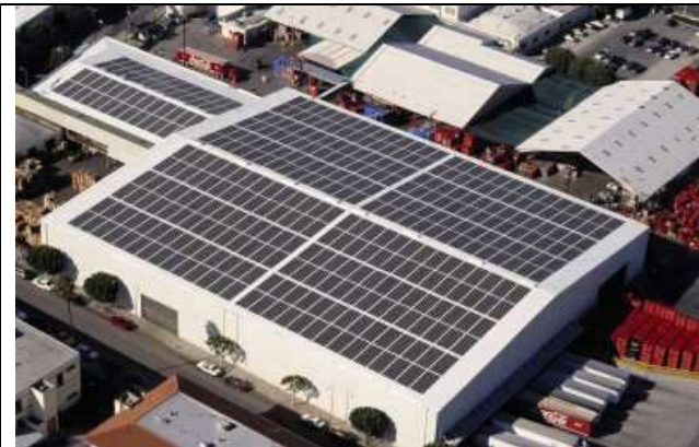
Fig. 5.18: PV Modules on top of an existing roof
