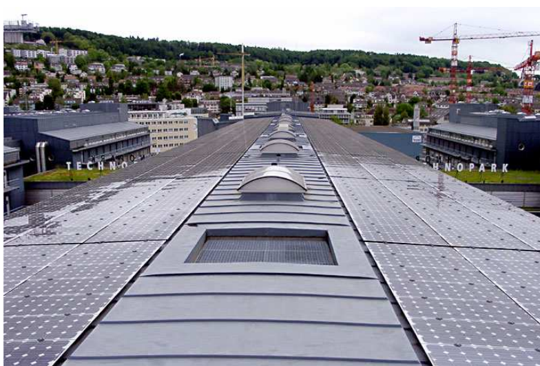
Fig. 5.13: Double roof at quasi-horizontal mounting of rimless PV modules (note the utilisation of the whole roof for PV module mounting) [53]
