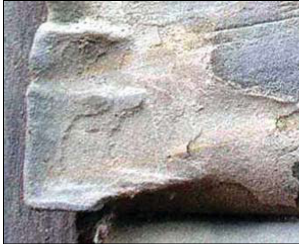
Figure 2.2: Granular disintegration and flaking of stone induced by salt crystallization (from ICOMOS-ISCS, 2008).
