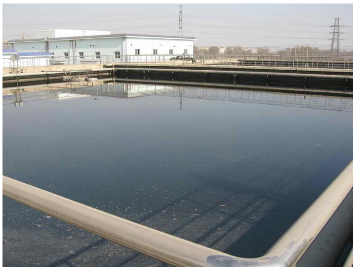
Figure 6-18: The SBR Basins in Wastewater treatment Plant (16.01.2011)
