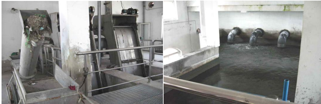
Figure 6-16: The coarse grid and promote pump station (16.01.2011)
