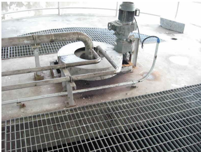
Figure 6-17: The pump in vortex grit chamber (16.01.2011)
