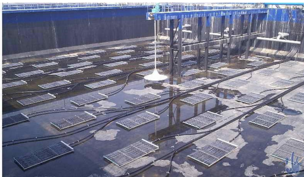
Figure 6-15: The plate-like aerators in SBR basin in Wastewater Treatment Plant of Old District
