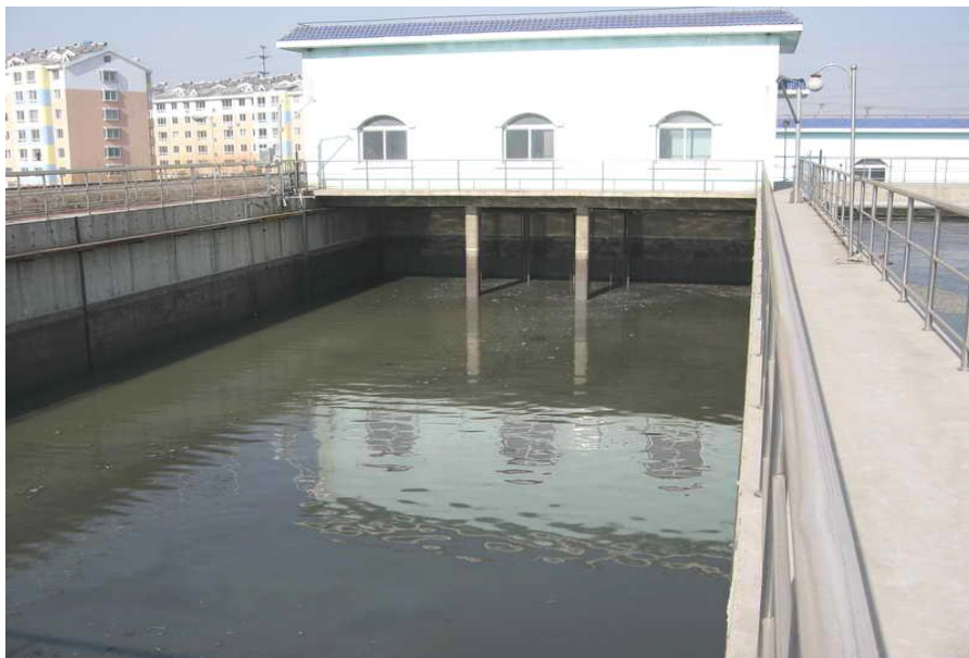
Figure 6-13: The pre-equalization tank in Wastewater Treatment Plant of New District (16.01.2011)
