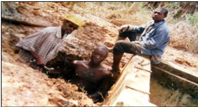
Picture 6.3 Community members employed and learning about plumbing services on-the-job Source: Accessed from the WSDB library in 2010
