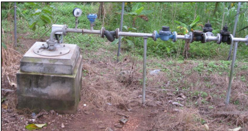
Picture 6.1 Submerged pump that feeds the ground level tank. Source: Author, 2010
