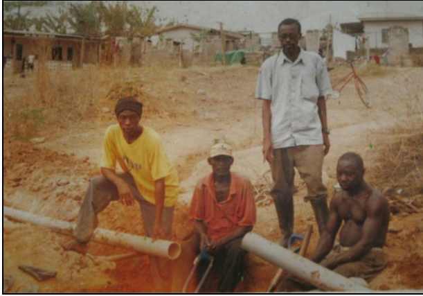
Picture 6.2 Community members employed and learning on-the-job about pipe-laying Source: Accessed from the WSDB library in 2010
