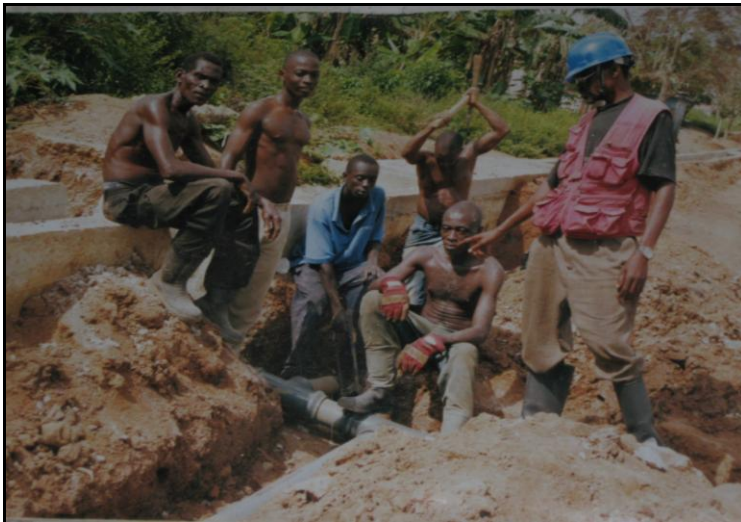
Picture 6.4 On-the-job training for security men and pump attendants organised by the WSDB Source: WSDB. Obtained during interviews conducted in 2010
