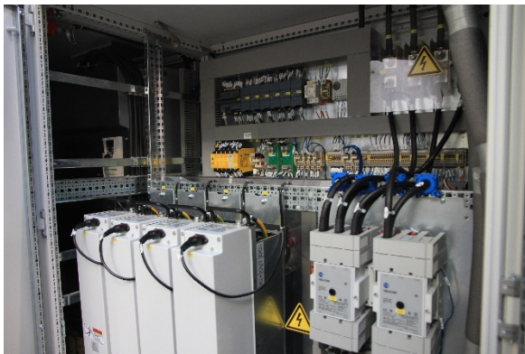
Power Amplifier System
