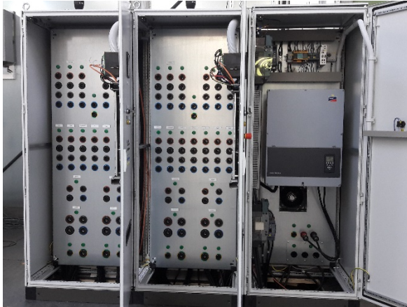
PV-Inverter connected to the busbar system
