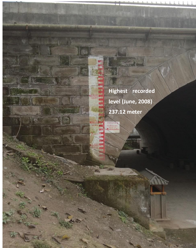
Figure 8.18 Water line on a bridge across Daxi River in Taojia town center.
